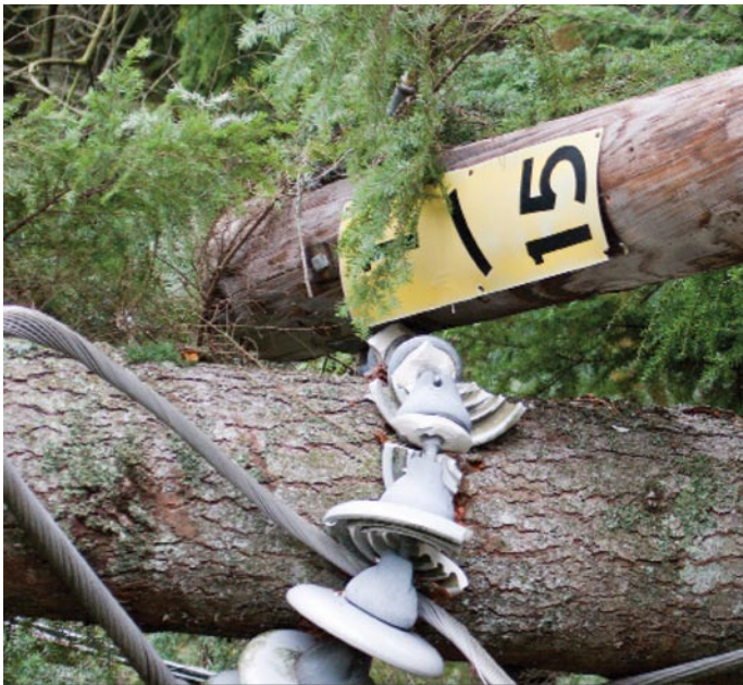
Trees and power lines can be a deadly combination. If you happen to come across a tree limb that has grown into power lines or fallen across them, contact Clark Electric Cooperative immediately.
